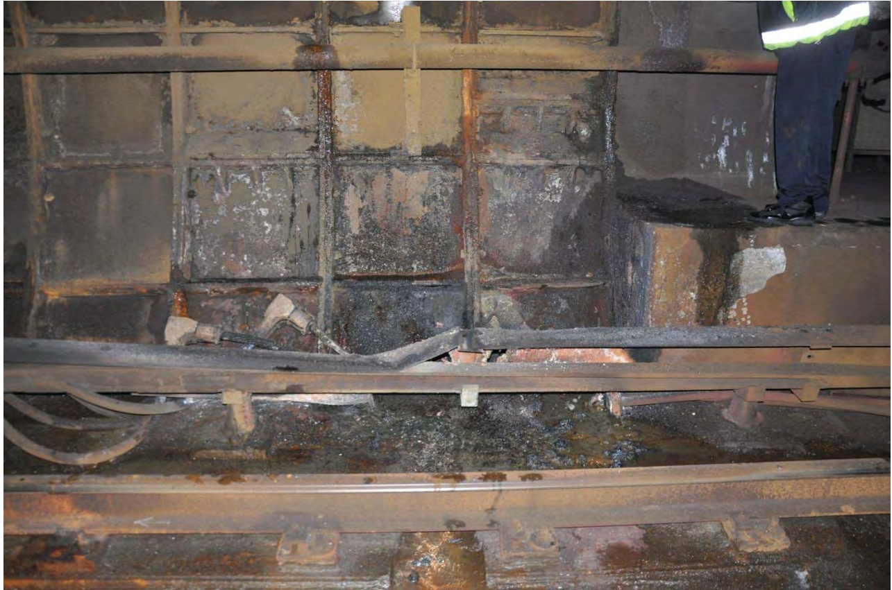
Figure 2. Damage from the arcing incident in the tunnel near L'Enfant Plaza Station.
