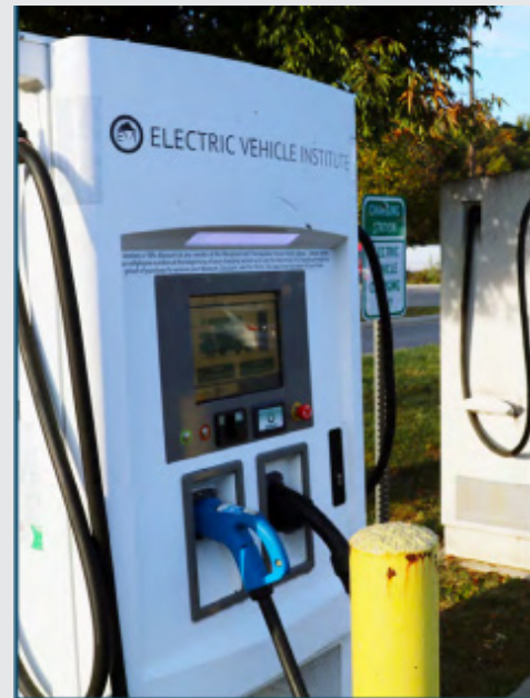
Figure 13: EV charging station (MDOT).
