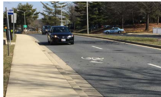
Faded shared lane markings on Girard Street approaching East Diamond Avenue
