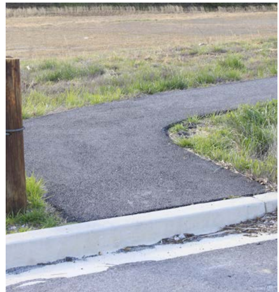
Path from MARC station to Parklands development missing curb ramp
