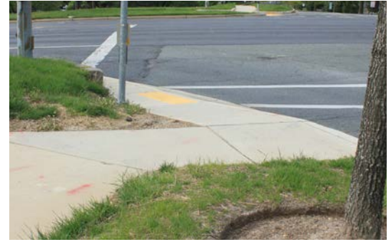
Steep slopes down to intersections are uncomfortable and unsafe for those in wheelchairs
