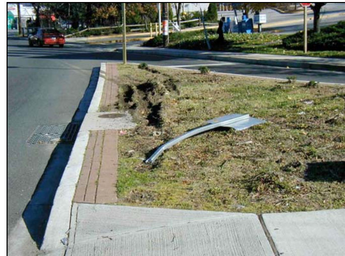
Figure 16: Recent Crash Remnants
